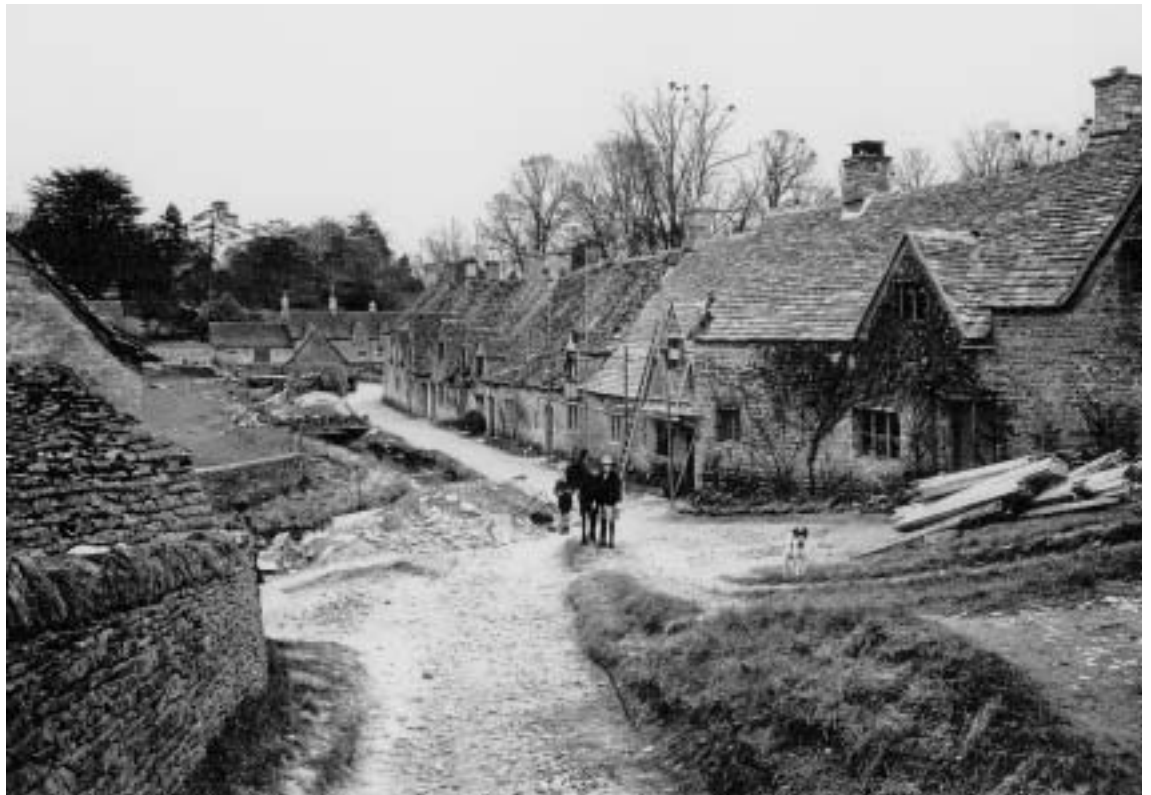
In this photograph, from the turn of the century, the stone slate roofs of Arlington Row are being repaired. These cottages have evolved over centuries - there have even been some minor changes since this photograph was taken.
