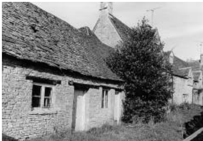
Two of the listed buildings in Bibury found to be in such poor condition as to be considered 'Buildings at Risk'. The Council will seek the proper repair of these buildings.
