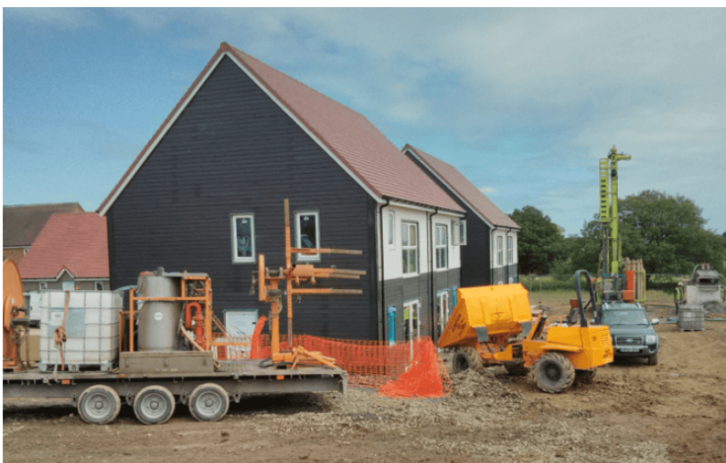
Figure 7 Installation of a shared ground loop array for ground source heat pumps in new build social housing
