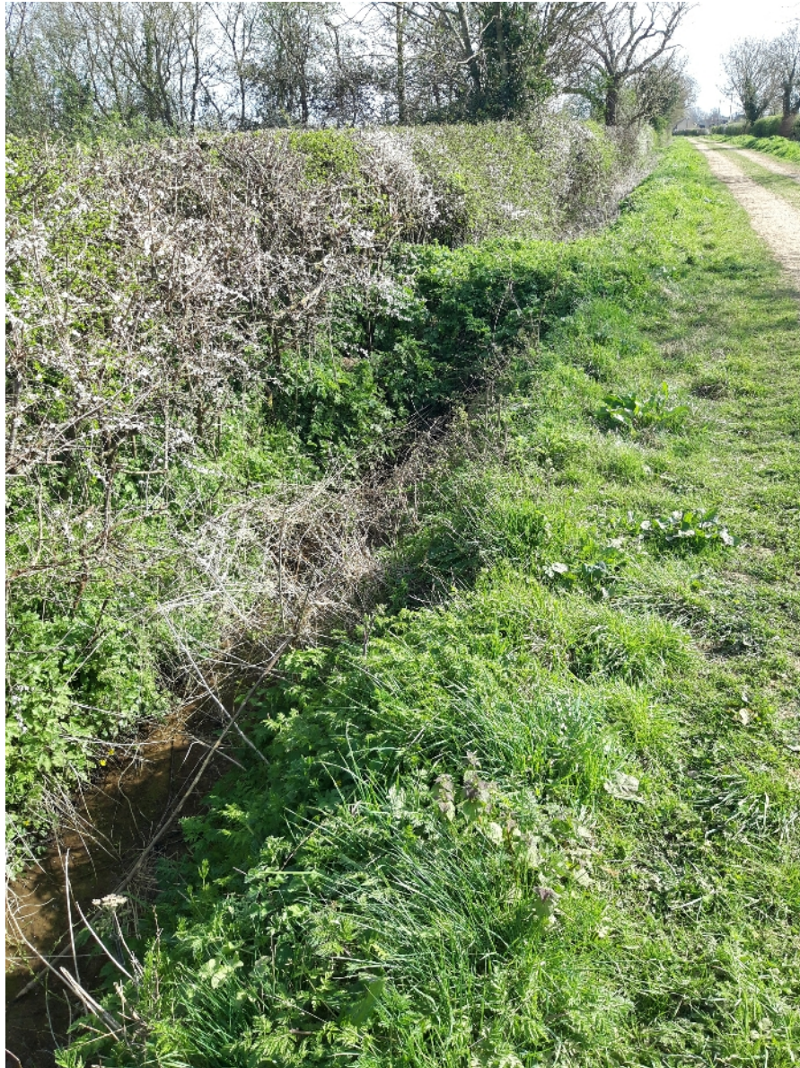
Photograph 2 – Drain B1 looking south showing obstruction
